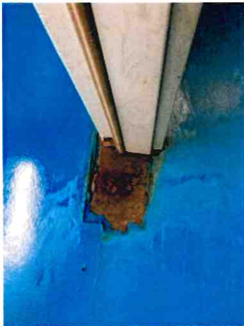
Portions of the floor have exposed/unsealed concrete
