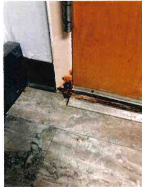
Portions of the door frames are corroded and repair or replacement
