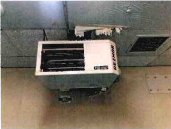
The HVAC system is exposed in the room
