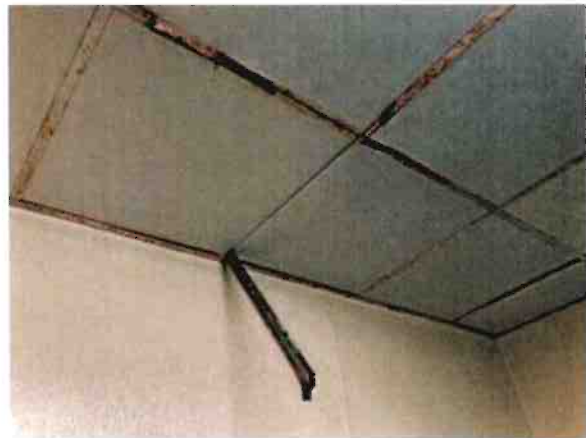
Ceiling system is corroded and needs repair or replacement
