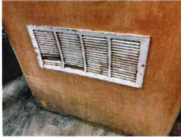
Air vents are rusted and deteriorating
