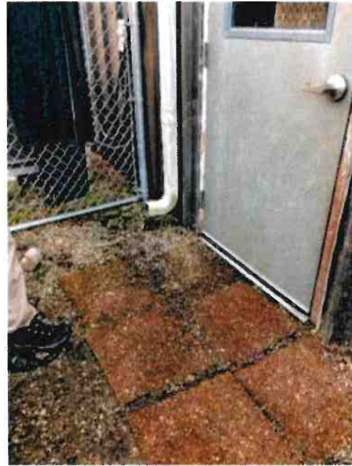
The downspout discharges water at the landing outside the backdoor of the dog kennels and water stands at the door landing after rain
