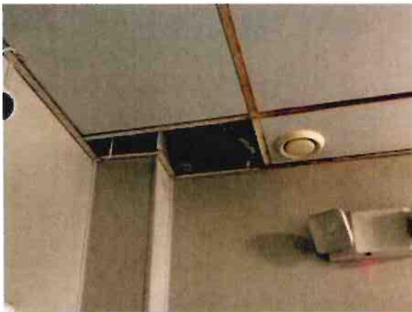
Ceiling system is missing tiles
