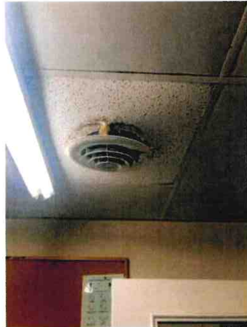
HVAC air device has dropped down from the ceiling
