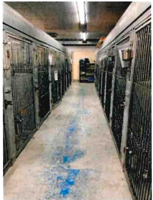
The ceiling in these dog kennels offers no sound absorption and the room is extremely loud
