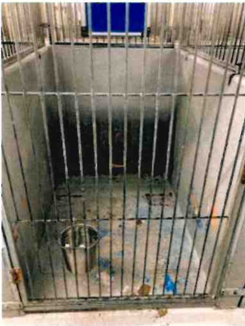
The dog kennels only provide single compartment housing. Furthermore, the finish is peeling off in many locations
